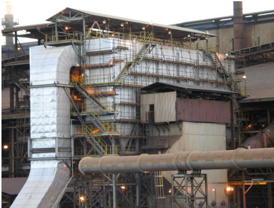
Figure 1 – New EF3 baghouse at PT Inco
