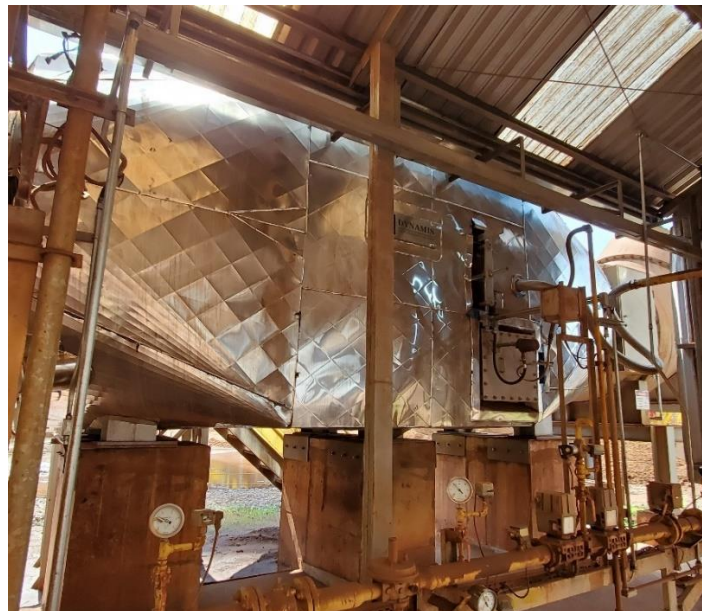
Fig. 3. Pellet Dryer Hot Gas Generator
