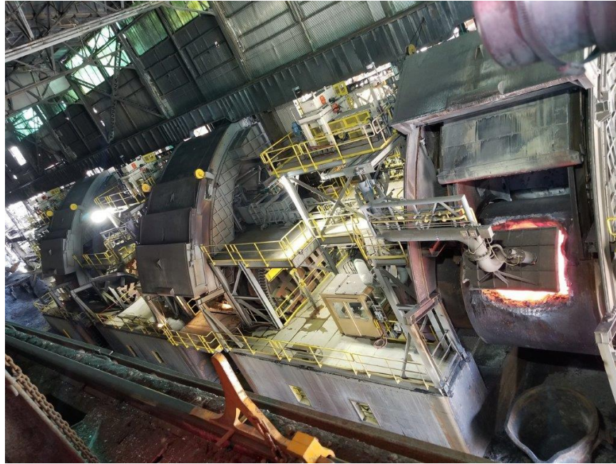
Figure 2. Converter Retrofit Project – Converter Aisle
