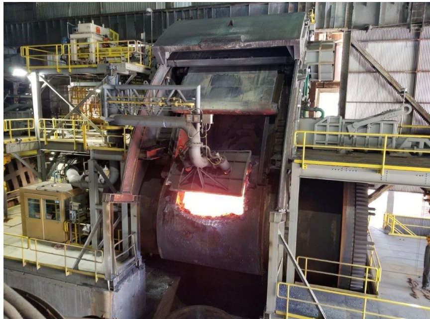
Figure 1. Converter Retrofit Project – New Converter and Hoods
